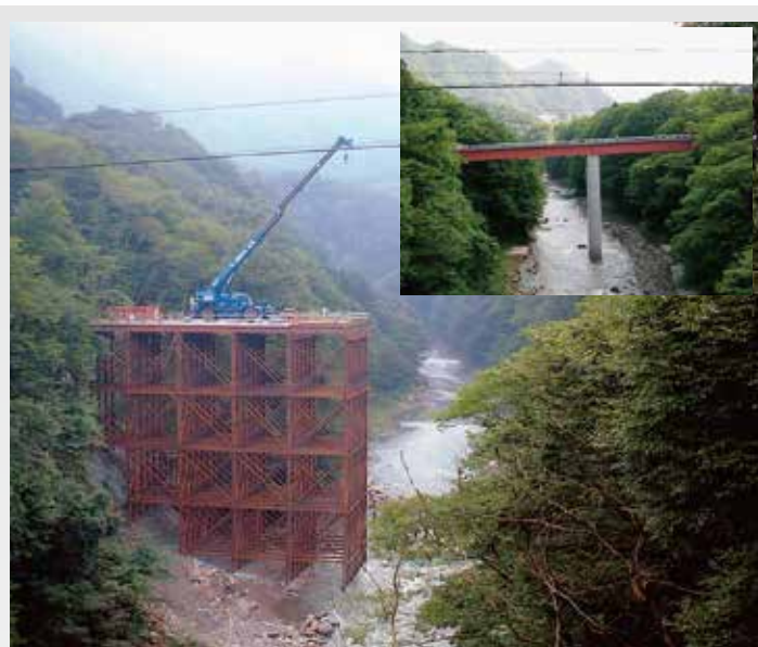
H400*400(support piles) L=7.5M~33.0Mx56 Setting pier construction 588m 2 Crawler crane 80t(suspension type) RX-2000(0.7m 3 )
